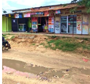
Plate 4.14: an improvised retail shops and a dry cleaner on a boundary wall, along a dilapidated access roads in Sinza "A", Source: Author, (2024).
