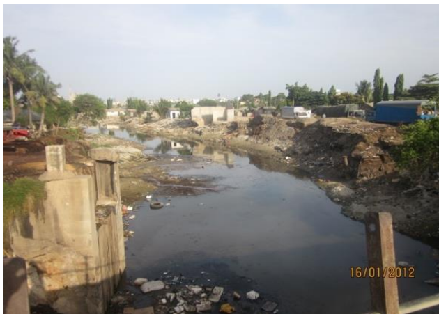
Image 6.1. Comparative flood impact showing protected and unprotected riverbank sections. Source: Field survey. (2025)
