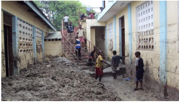
Image 3.5. Flood damage observed within Luhanga Catholic Church premises. Source: Field survey (2025)
