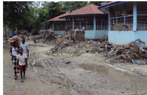
Image 3.10. Flood impacts on Gonzaga Primary walkways. Source: Field survey (2025)
